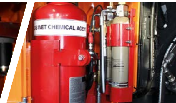
Automatic fire-extinguishing system
