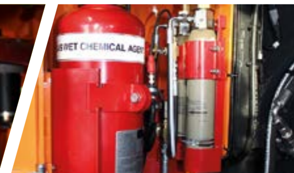
Automatic fire suppression system
