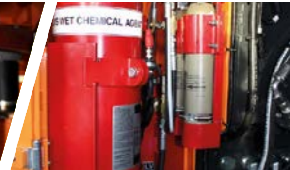
Automatic fire suppression system
