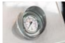
External pressure control Gauge
